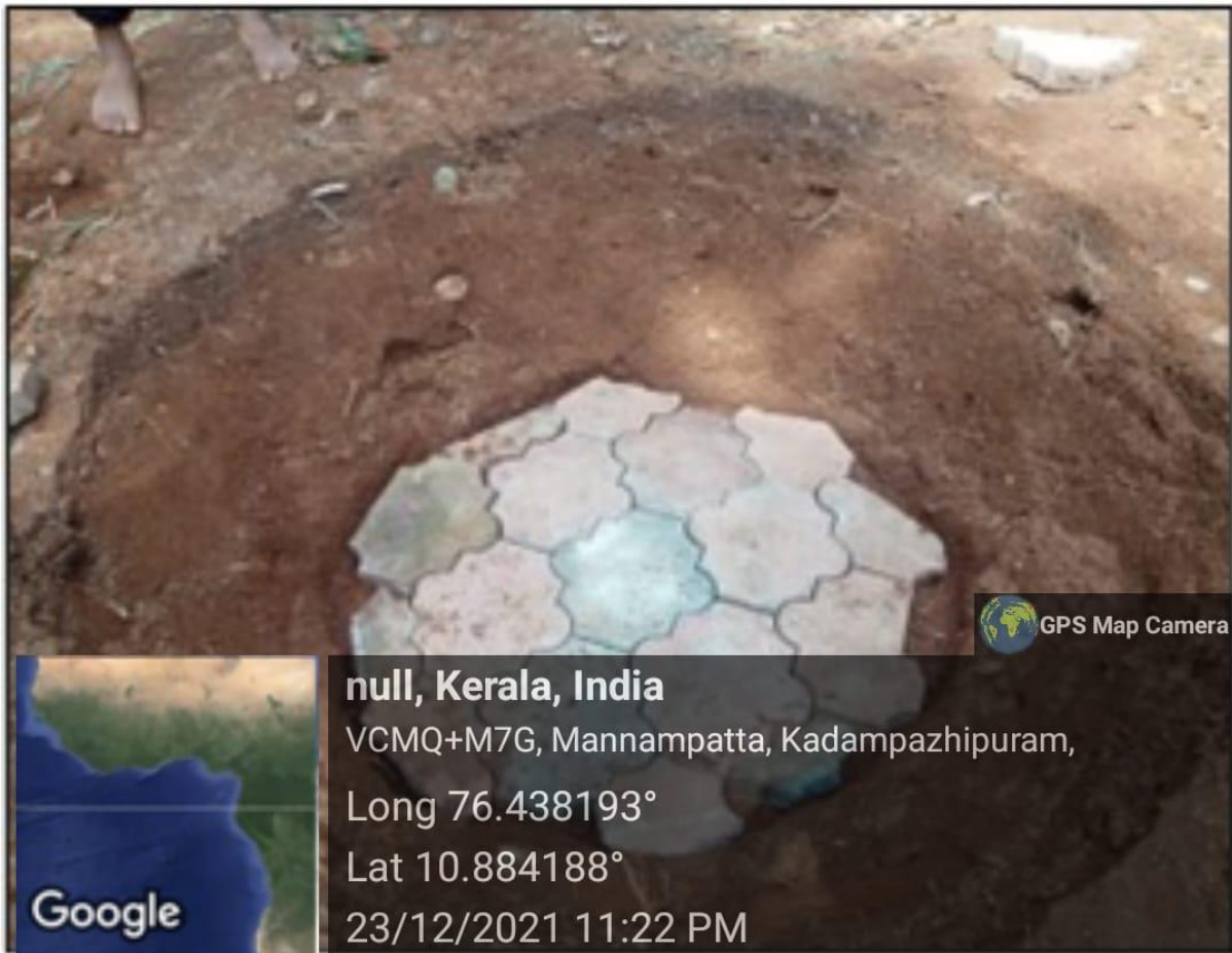
On 23/12/2021, the interior of the Water Lily Pond is leveled using interlock tiles.
